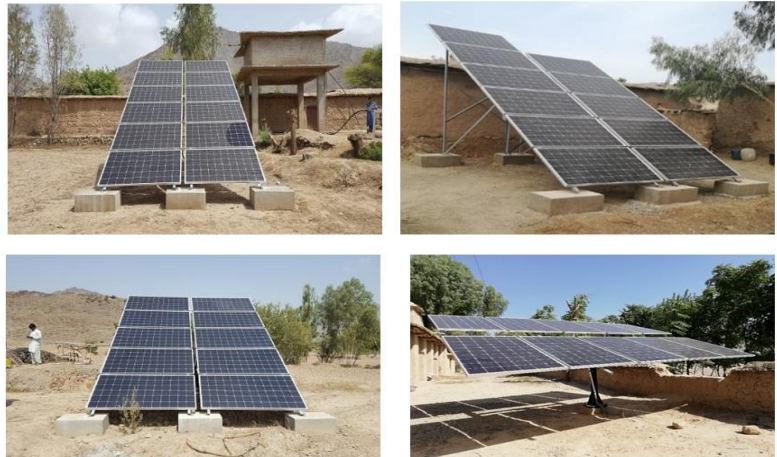
Solar Pumping Projects at FATA Newly merged Area (Mohmand)
