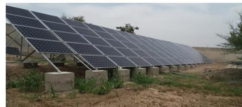
Solar pumping project at Karak
